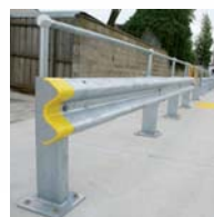
W-Beam Guard Fence
